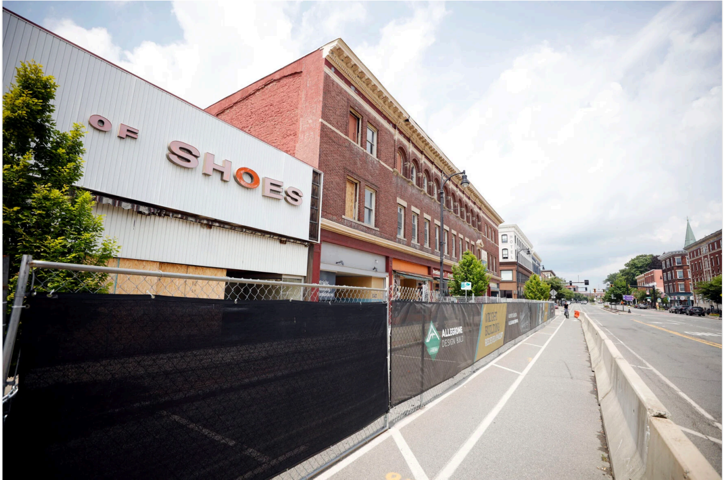
The Wright Building redevelopment is on track to welcome tenants next year thanks to $4 million from the state
