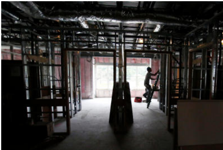
Work continues on Berkshire Place on South Street in Pittsfield. Allegrone, the company in charge of the project, aims to finish construction in October.
